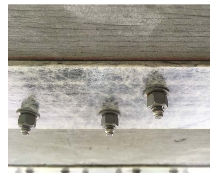
Close-up of the FRP strips on the underside of a bent on bridge 98 on I-89 in Swanton
