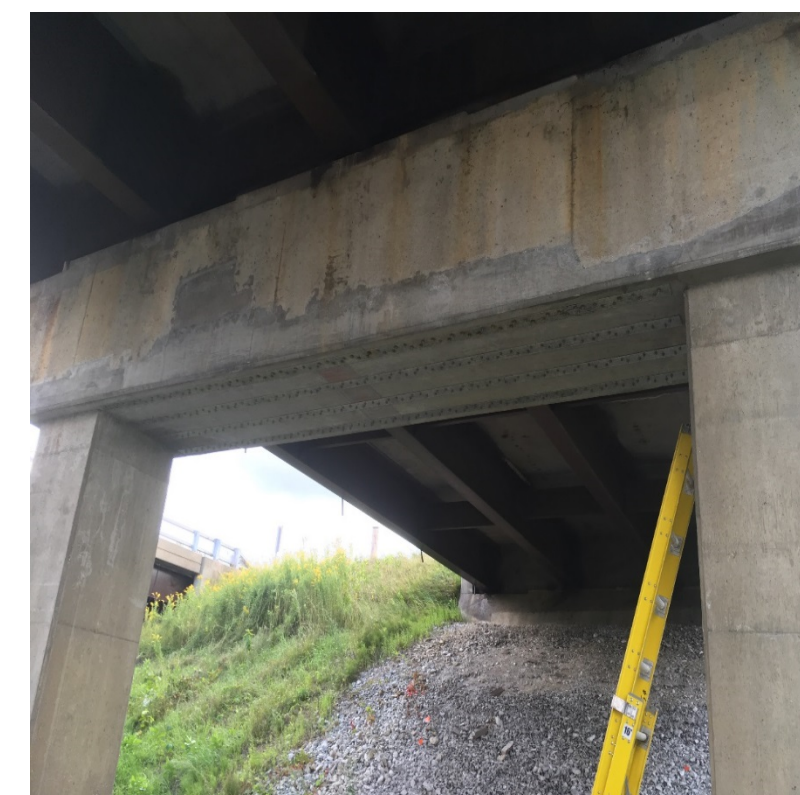
Fiber Reinforced Polymer (FRP) strips on the underside of a bent on bridge 98 on I-89 in Swanton
