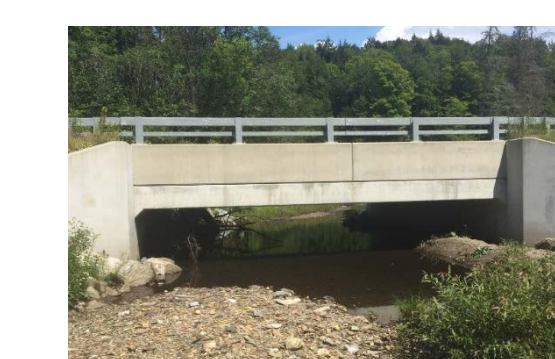
BDM system, Bridge 165 on Route 100 in Warren
